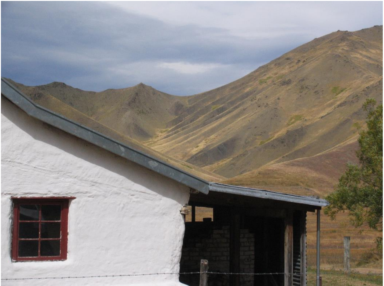
The recently renovated Cob Cottage at the Acheron and Clarence confluence, Molesworth Station
